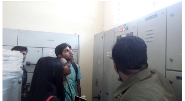
Final Year Electrical Students at power distribution panel, BMSIT&M Campus.
